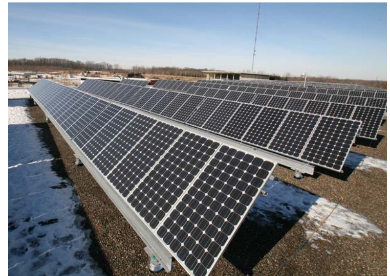
Solar panels on the roof of Hennepin County Public Works Facility in Medina.
