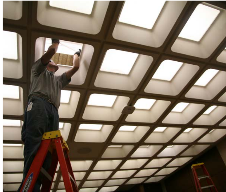
Replacing the lighting at the Hennepin County Government Center with an energy-efficient option
