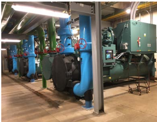
Capital project in 2017 to replace electric chillers at the Hennepin County Energy Center with more efficient models, saving $175,000 per year in electricity costs.
